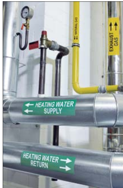
Large and highly visible pipe marking.
